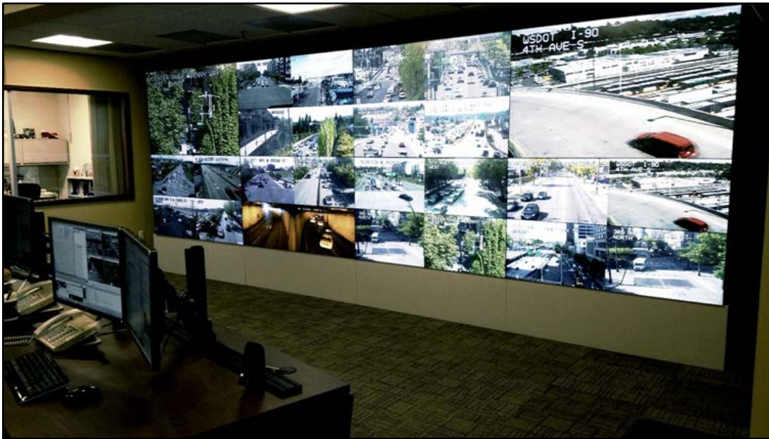
Figure 4: SDOT Transportation Operations Center
