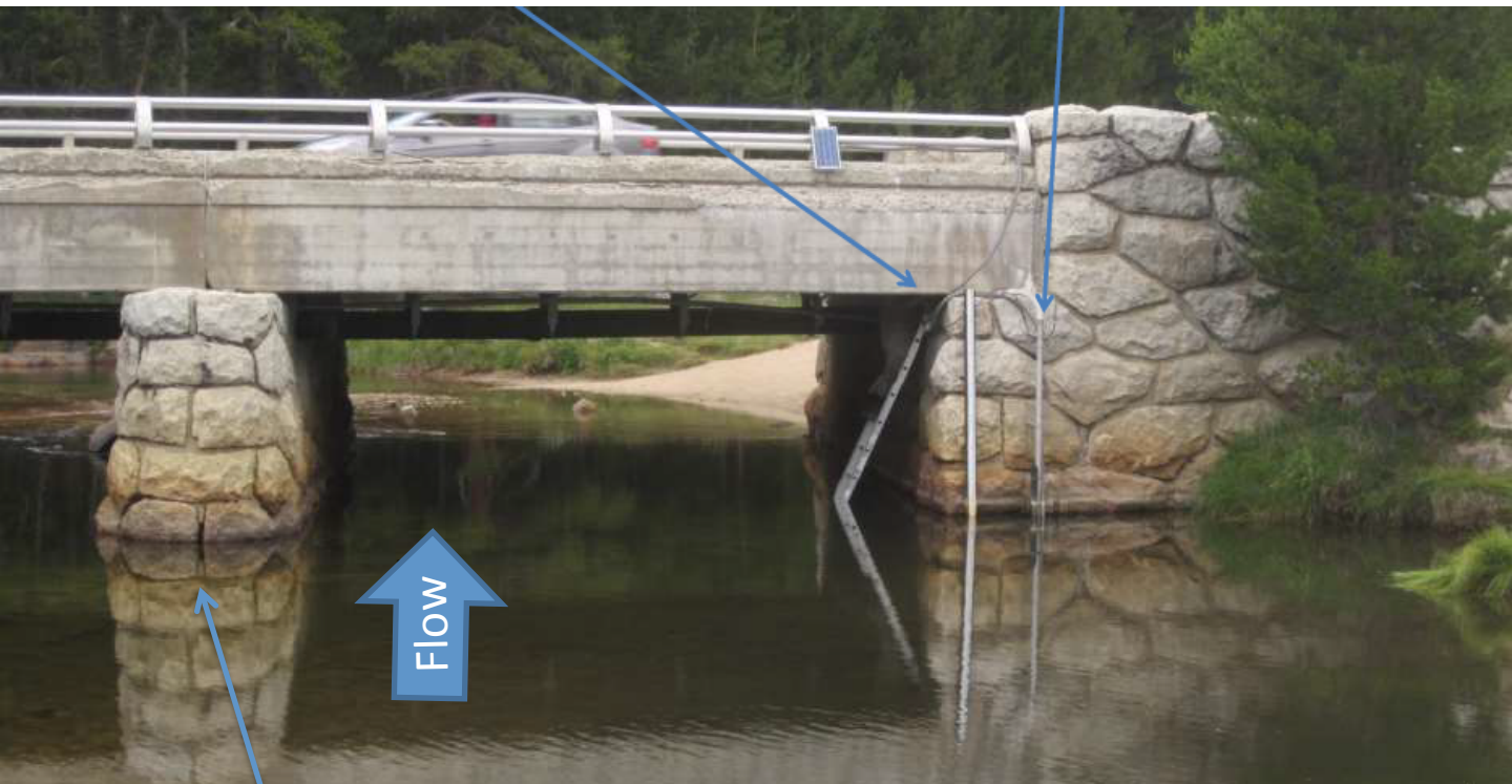
Original install in 2001, anchored solinst at the base of this abutment.
