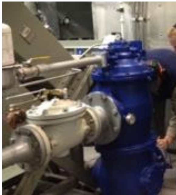
Figure 1.3 Self-cleaning filter installed on M/V Chetzemoka
