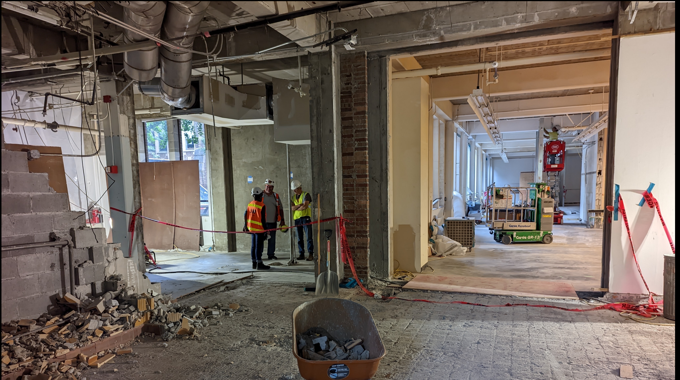
Entryway, “window” into Advanced Concepts Lab and Woodshop, and adjacent spaces towards new Jacob Lawrence Gallery
