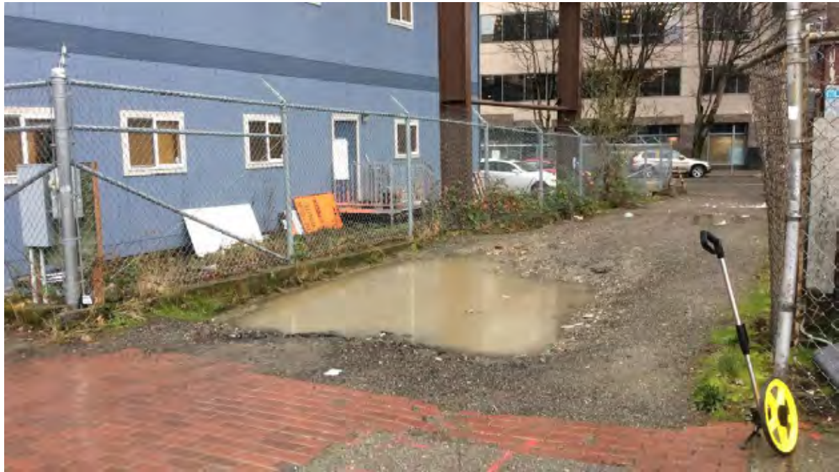
Figures 1-7, 1-8, 1-9, 1-10. Examples of Center City Area Alleys with Poor Pavement Condition for Loaded Handcarts
