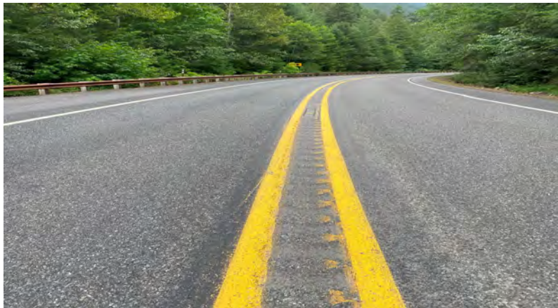
Figure 4-32. Photo. Condition of SR 20 in Summer 2023.
