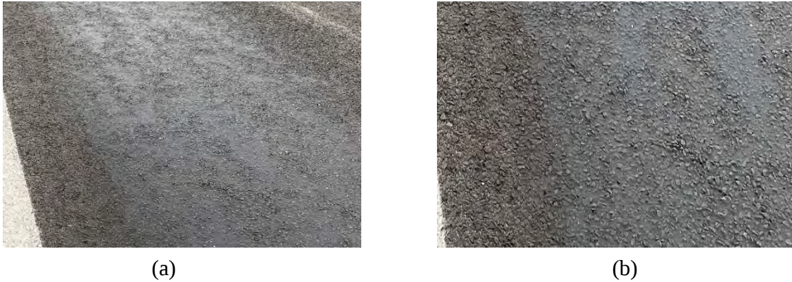
Figure 3-9. Photo. US 195 (a) Bleeding in the Wheelpath, and (b) Close-up View with Chips.
