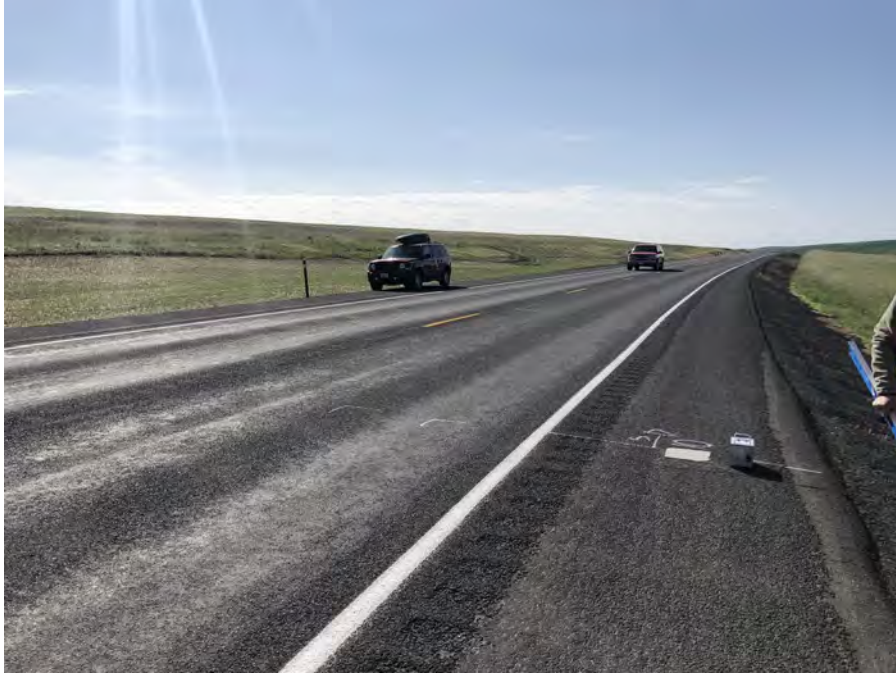
Figure 4-15. Photo. Bleeding Issues on US 195.
