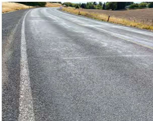
Figure 4-13. Photo. Condition of SR 27 in Summer 2023.
