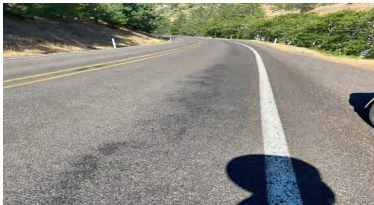
Figure 4-37. Photo. Slight Bleeding of SR 142.
