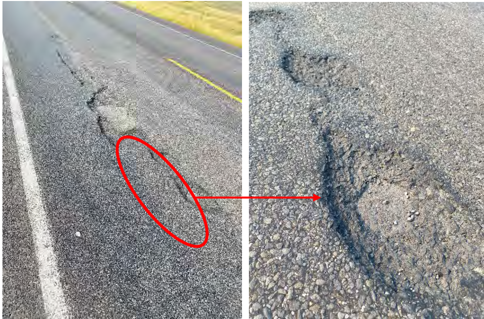
Figure 4-21. Photo. US 195 Extensive Blowup Under the Wheelpath.
