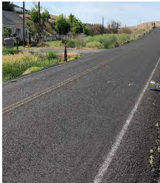
Figure 4-23. Photo. Condition of SR 261 in Summer 2023.
