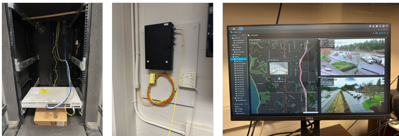
Figure 5-15 CCTV access directly at the UW STAR Lab (Mar 20, 2025).
