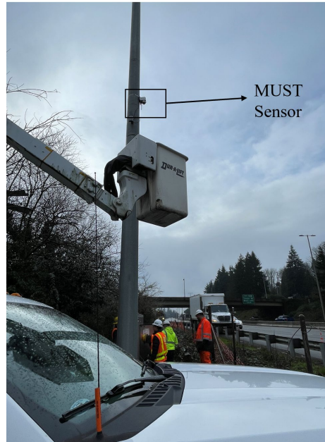
Figure 11. The installed MUST sensor.
