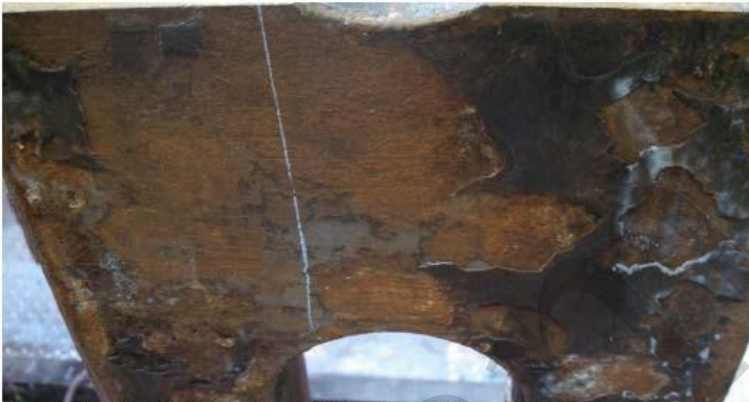
Fig. 1. Crack noted in bottom of 3A plate at X end
